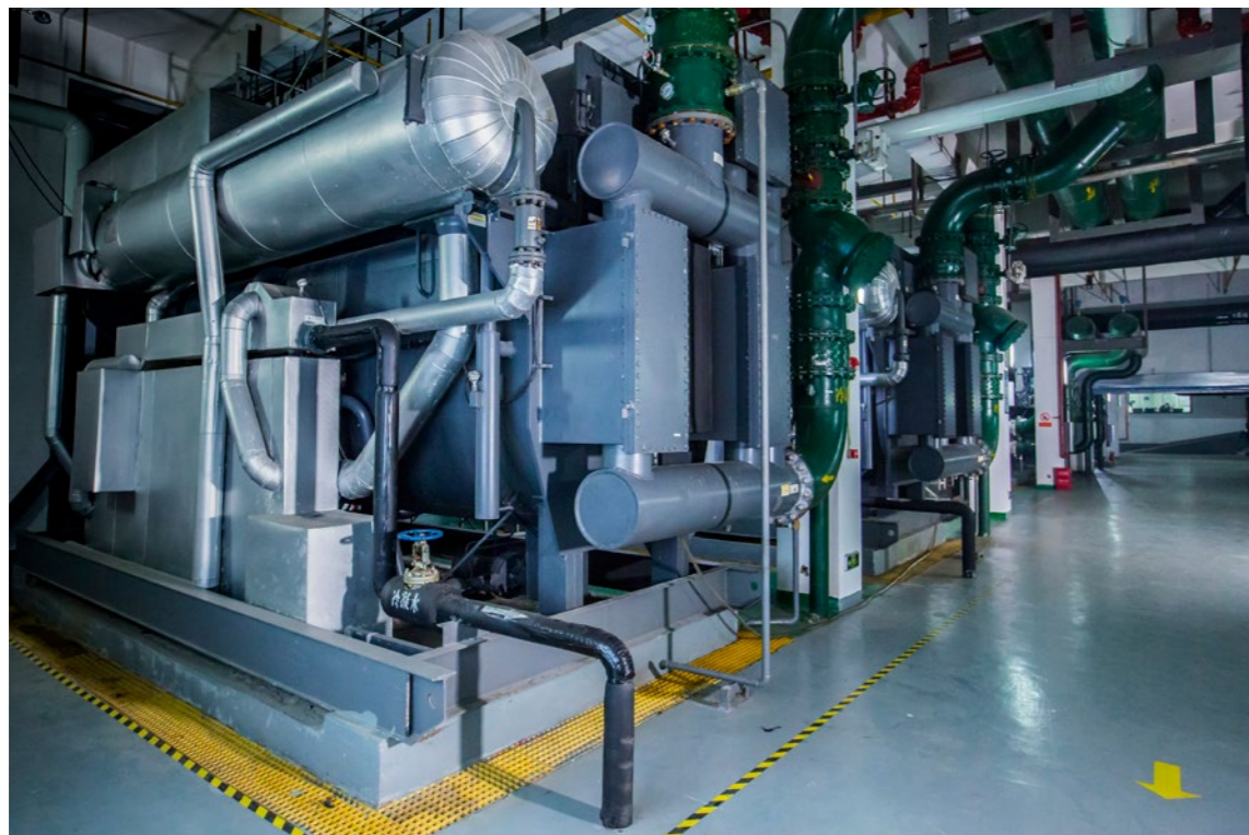
CEC Energy-saving Financial Harbor – energy station
